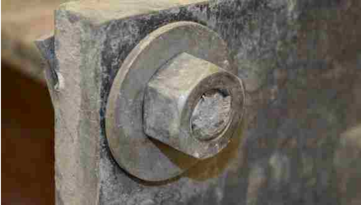
Figure 4-14: Broken Anchor Bolt
